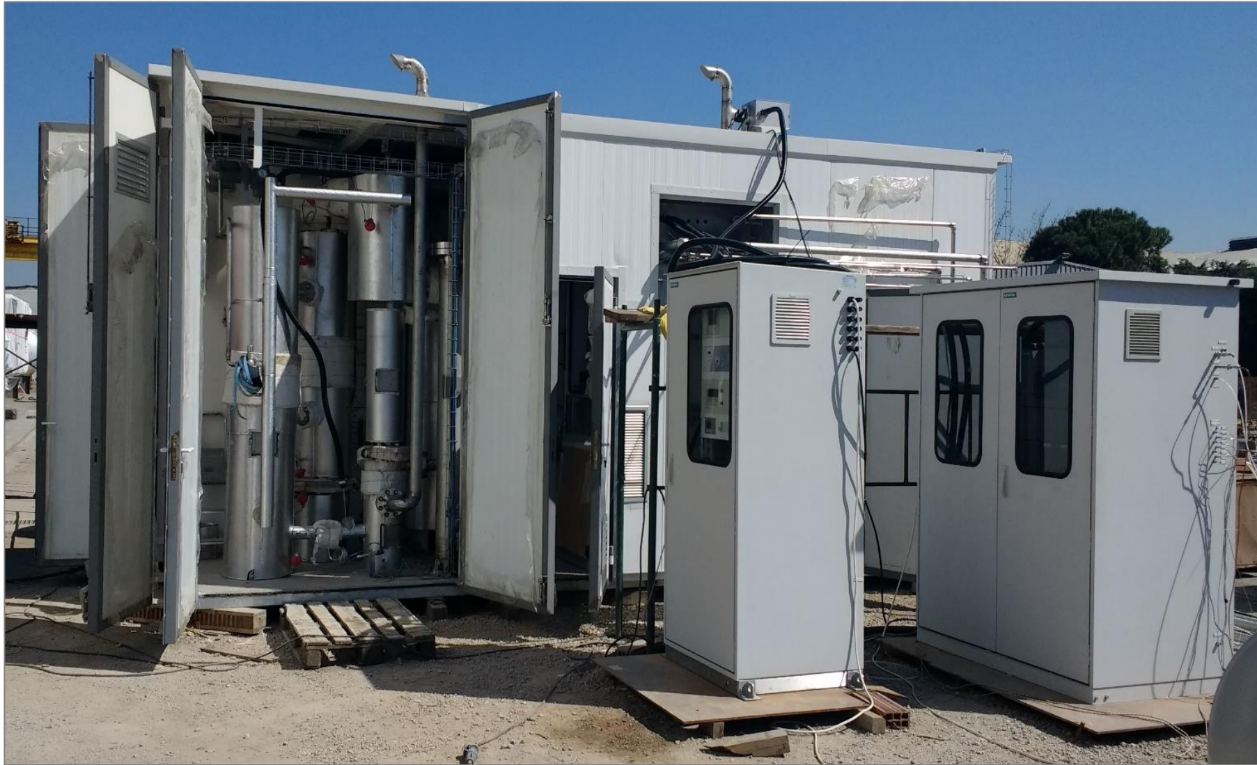
Hydrogen generator process & gas analysis system
