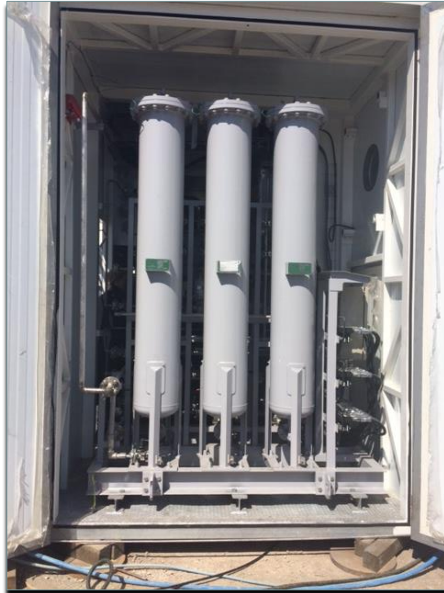
PSA (Pressure Swing Adsorption), hydrogen purification system
